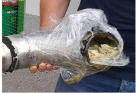
Ammonia carbamate formed in a pipe
