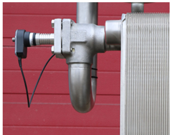
HBX sensor in strainer housing used as leakage detector installed after plate heat exchanger
