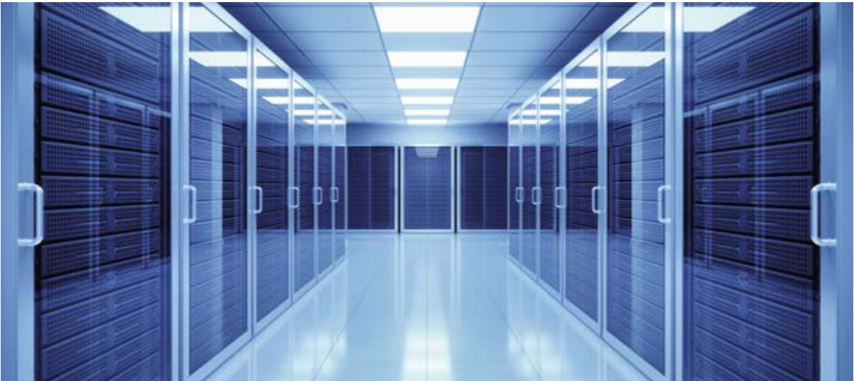
Data centre cooling
