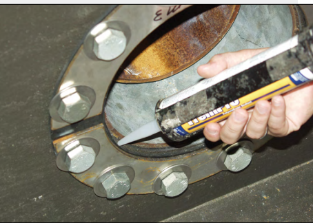
Figure 13. Caulk Exposed Galvanized Steel
